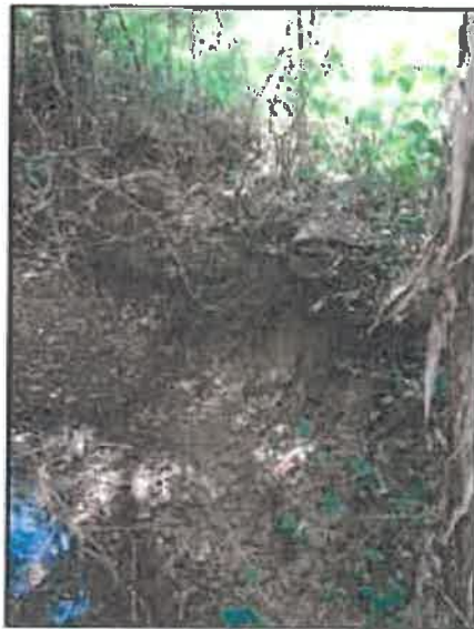
Evidence of trash and debris (55-gallon drum) in the stream at the proposed crossing
